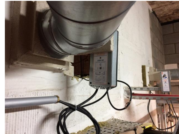
Example of excessive Builders Work Holes.
