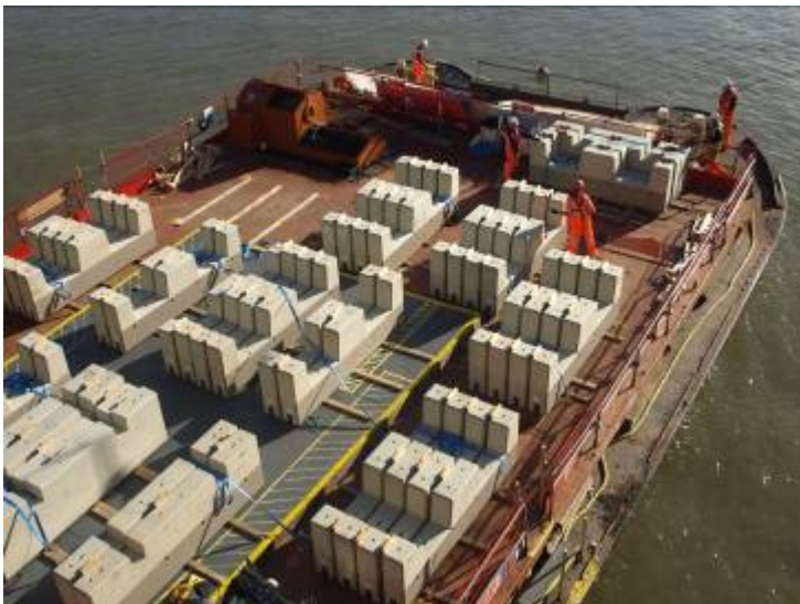
Photograph 1: Prefabricated platform units being delivered to the Blackfriars site via marine transport
