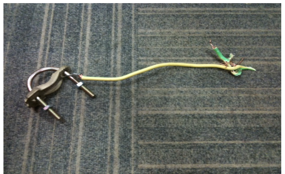
Example of broken bond / unauthorized removal of Bond
