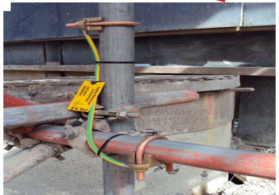
Earthing Bond with tag in place
