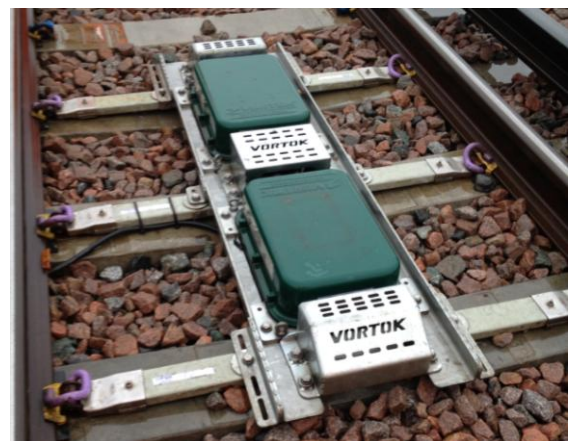
Figure 2: new design of AWS installed on TLP
