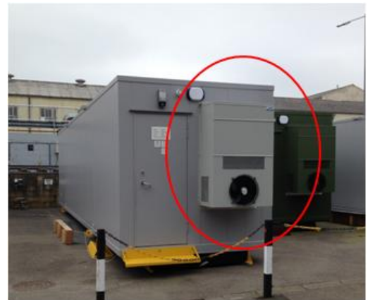
Figure 1. HVAC on REB
