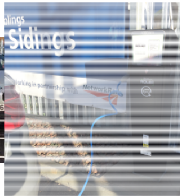
Photo 2 – Rolec EV charging point
