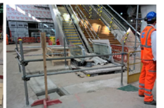
Scaffold with Key clamp fixings
