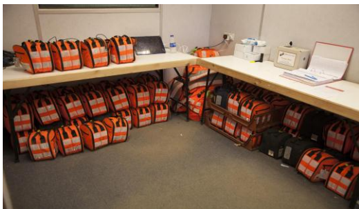
Interior of CSC at Gemini showing setup of communication system
