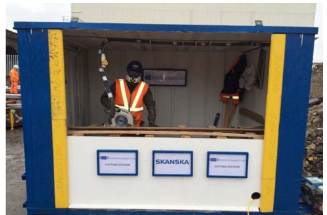
An operative at the BDU site utilising the cutting station wearing the half mask
