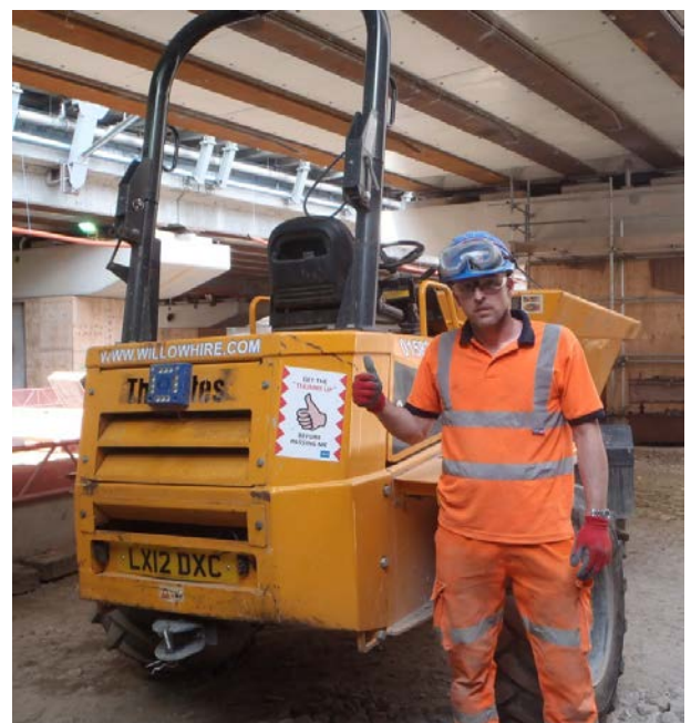
An operative at the Costain London Bridge site above demonstrating the positive response needed from plant operators before being allowed to pass.
